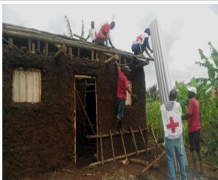
Shelter beneficiary being supported by volunteer to recover the house roofing during floods operation in Nyamasheke district. Photo RRC
