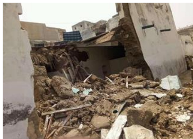
Picture 1: Hadramout, mud house affected by the flood. Photo: YRCS
