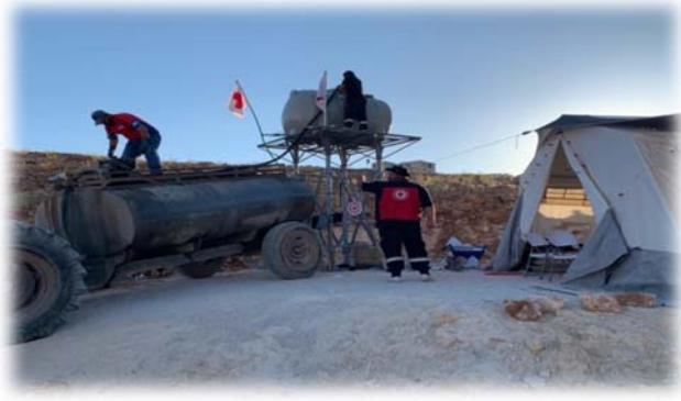
Figure 5. Water installation at Site Everest, Credit: LRC
