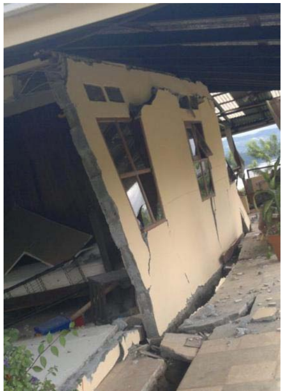
Damage and need assessments are still ongoing across Costa Rica to gather information on affected homes and buildings. Source: Costa Rican Red Cross.
