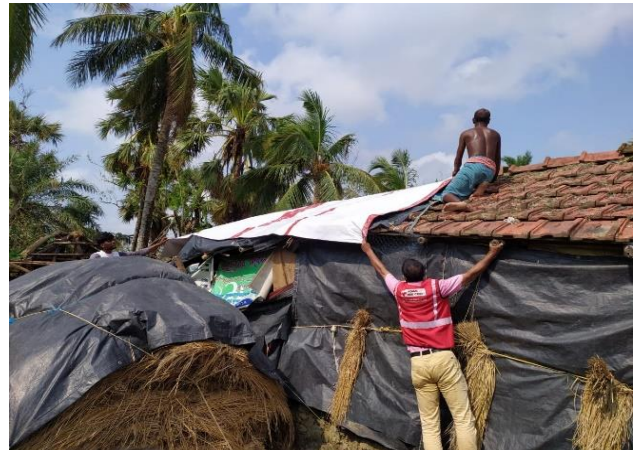
Indian Red Cross volunteer covering a broken hut in a cyclone affected community. (Photo: IRCS)
