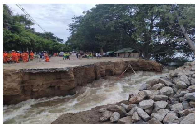
Collapsed river in Amarapura, Mandalay, with a geological sedimentary dike broken upstream, causing heavy flooding downstream. (Photo: MRCS Mandalay branch)
