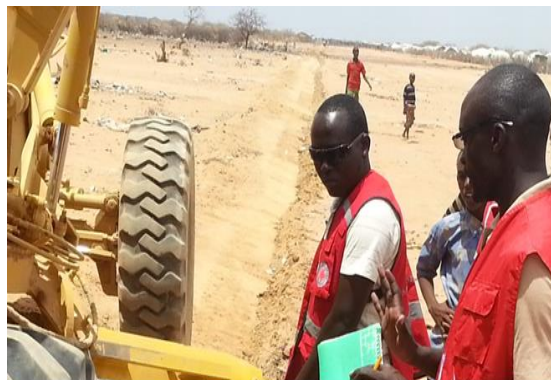
The KRCS technical team instructing the plant operator during trenching works in both Ifo 2 West and East. Photo / KRCS.
