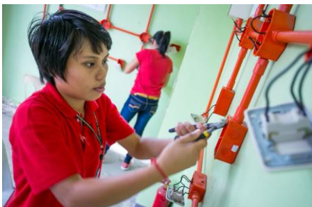
Maria Kristy Bacho, 19, from San Miguel, Leyte, enrolled in an electrical installation and maintenance course. Kristy's new qualifications will help her break into what has been a traditionally male-dominated industry.
