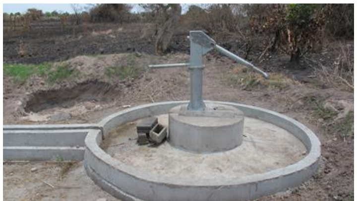
Five bore holes were constructed in Mudiba and 1 de Maio, Mopeia district. Photo by IFRC
