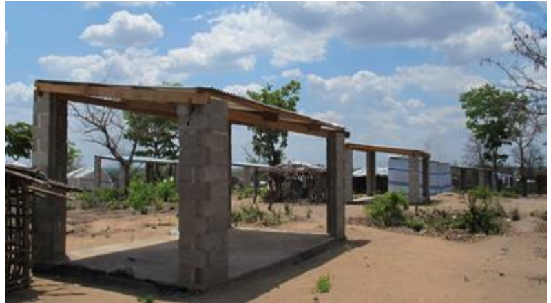
Current core structure which needs to be reinforced with two additional pillars. Photo by IFRC
