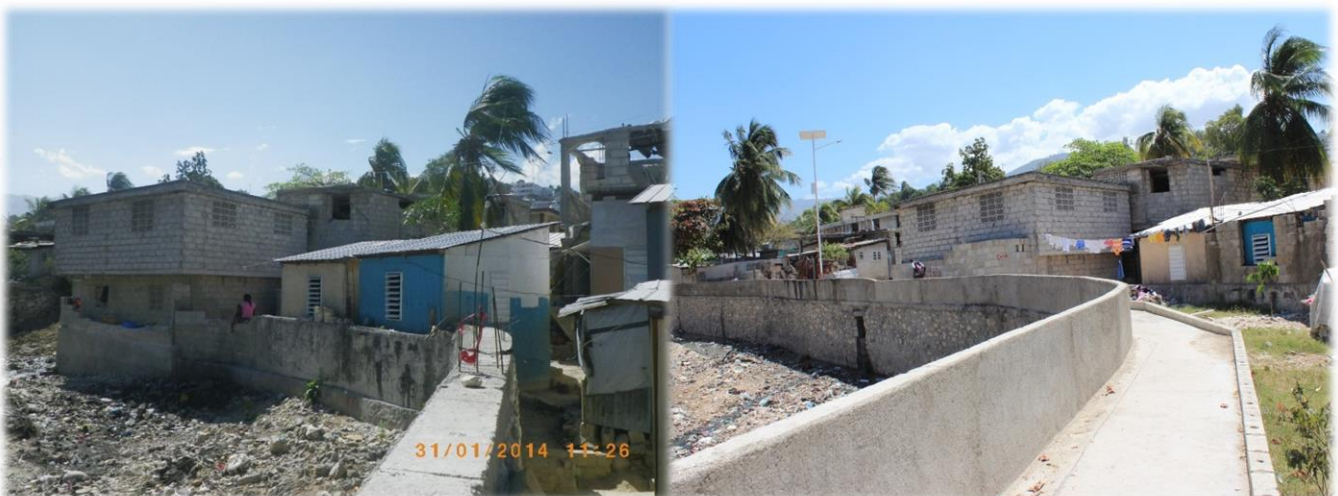
The Ravine rehabilitation work BEFORE and After as part of the implementation of the second phase of the Integrated Neighbourhood Approach programme in the Commune of Delmas 7, 9, 11 and 13.
