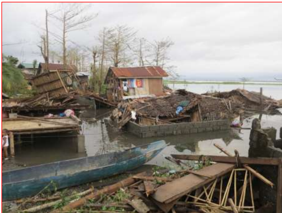
In the town of Najuan, province of Oriental Mindoro, hundreds of shelters made of light materials have been severely damaged or destroyed by both the strong winds and subsequent floods. Photo: Byron Nonato/IFRC
