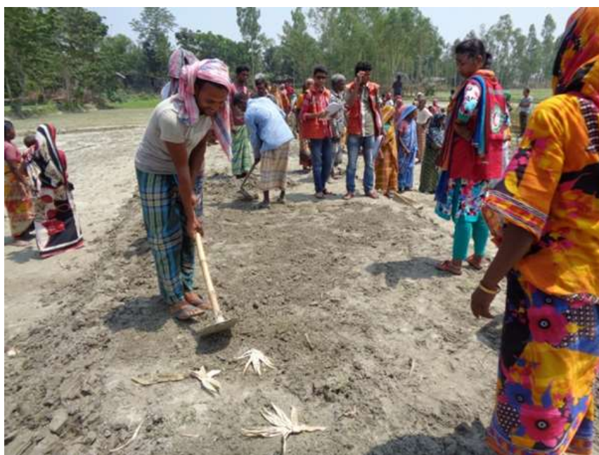
Cash for work to improve the road conditions in flood affected communities in Shirajganj district
