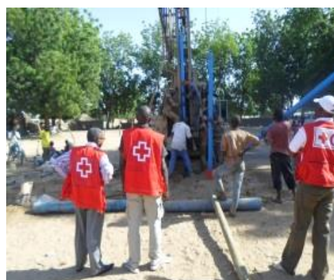
Construction workers installing a tube after drilling in Warba, under CRC and IFRC © IFRC.Photo CRC
