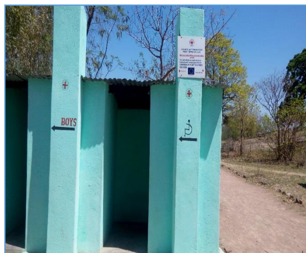
FIGURE 3.10: Disability friendly toilet at Mawadze School
