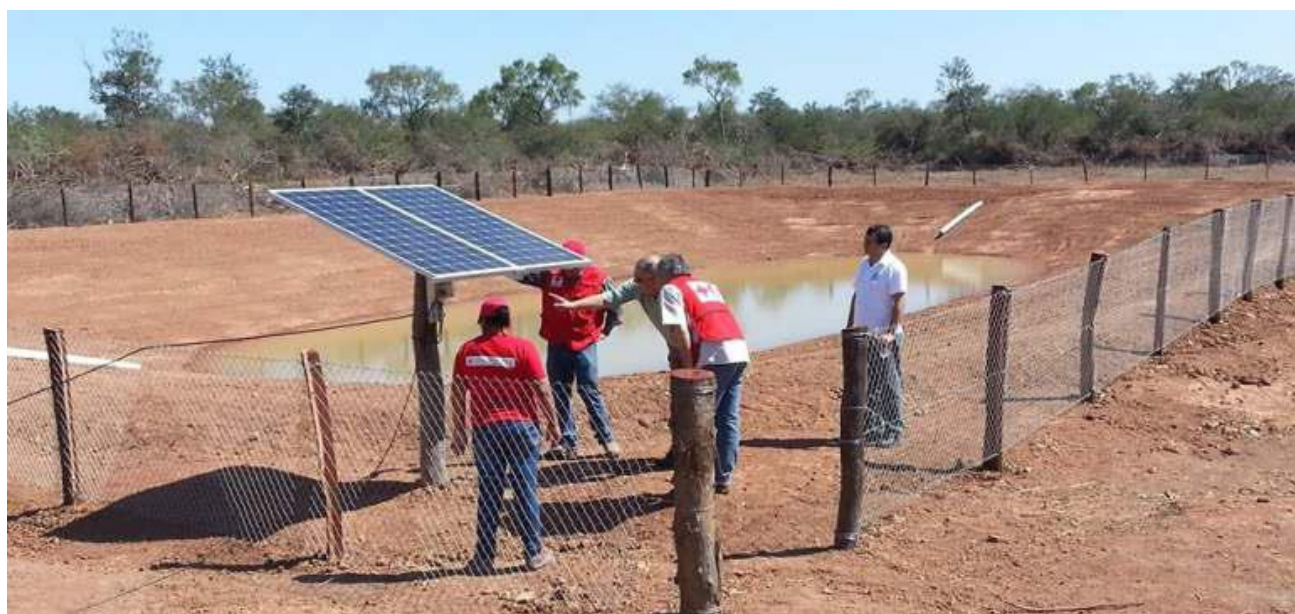
A 3000m 3 pond, pumping system ( tajamar ) with solar panel with closed perimeter built in the municipality of Filadelfia to improve water catchment capacity to support the sustainability of the families' livelihoods. Source: Paraguayan Red Cross.
