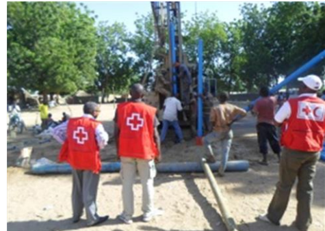
Construction workers installing a tube after drilling in Warba, under CRC and IFRC © IFRC
