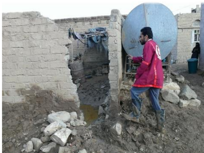
A YRCS Amran branch volunteer assessing damage caused by the heavy rainfall Source: YRCS
