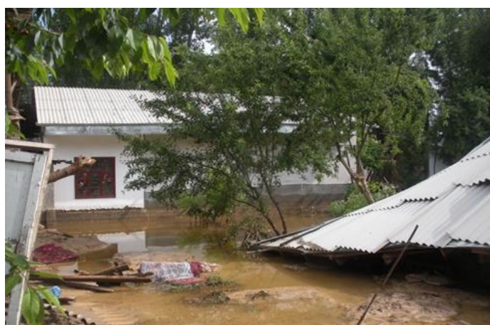
House destroyed in Panjekent district. Photo by: RCST Panjekent branch.
