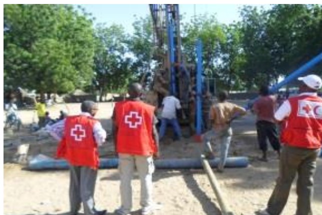
Construction workers installing a tube after drilling in Warba, under CRC and IFRC supervision © IFRC
