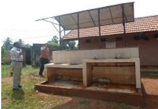
Poorly maintained water facility Kuddiyapulam – Thellippalai DS
