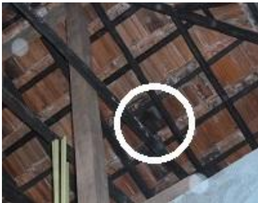
Roof timber and tiles properly connected, timber (circled) immature and tiles (circled) of poor quality
