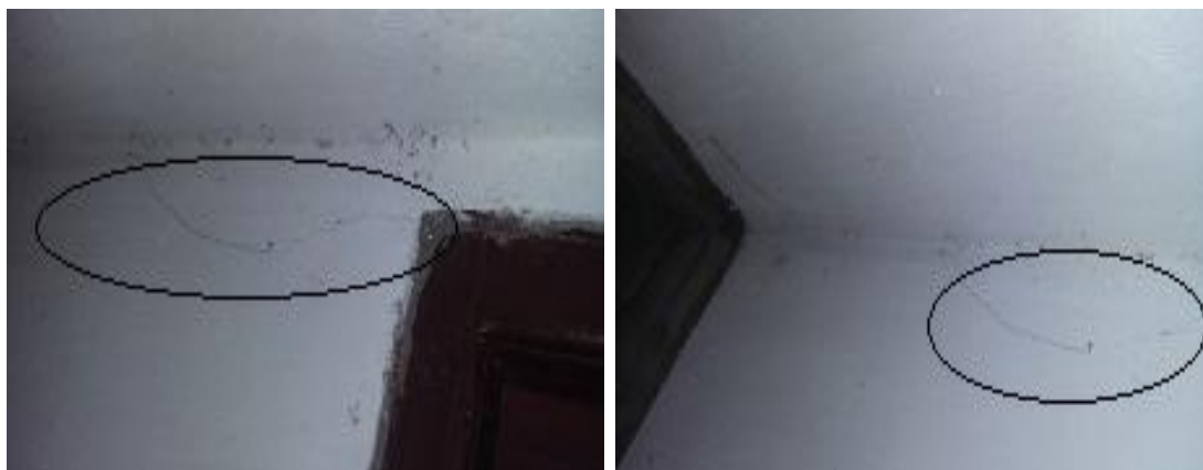
Sample of minor wall cracks
