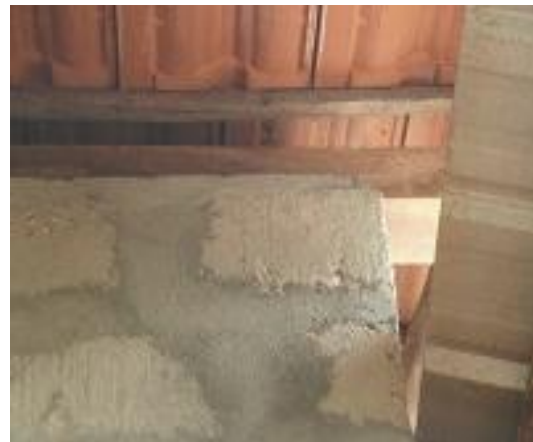
Roof timber not joined properly, no preservatives used and not anchored with the superstructure
