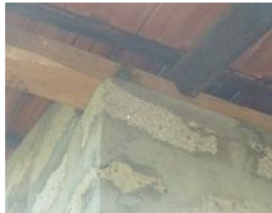
Roof properly connected anchored but not treated with preservatives
