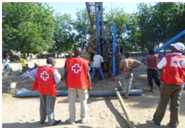
Construction workers installing a tube after drilling in Warba, under CRC and IFRC supervision © IFRC
