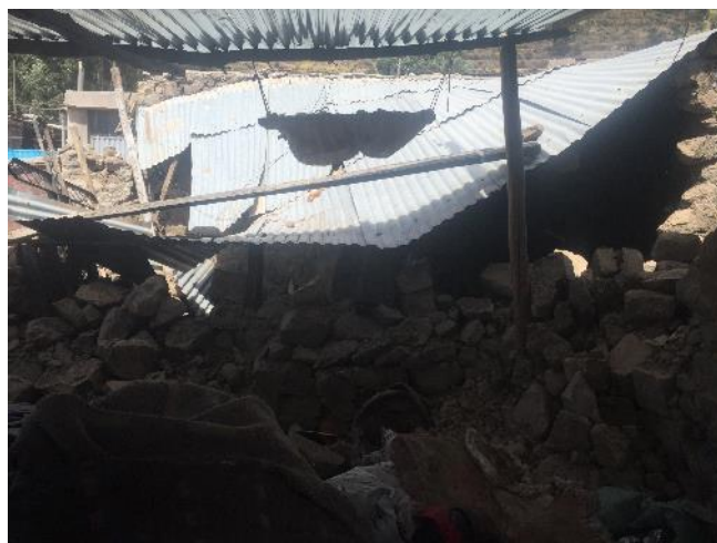
Collapsed houses in the city of Achome. Source: PRC
