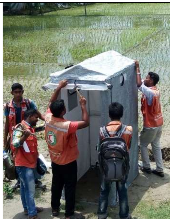
Volunteers are installing mobile latrine in Bogra District. Photo: Bogra RC unit/BDRCS
