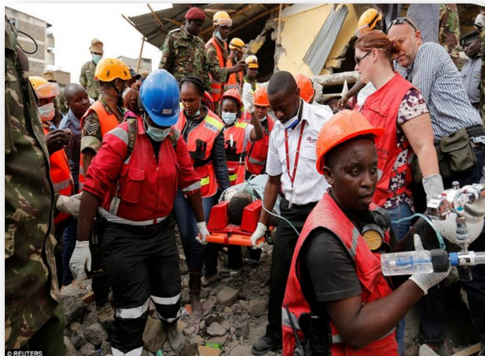
Figure 2: Search and rescue efforts with other partners at Huruma Collapsed Building. Photo KRCS
