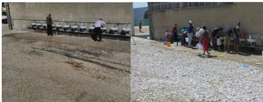
Before and after the drainage construction in the water points in Kordelio-Softex. Photo: IFRC
