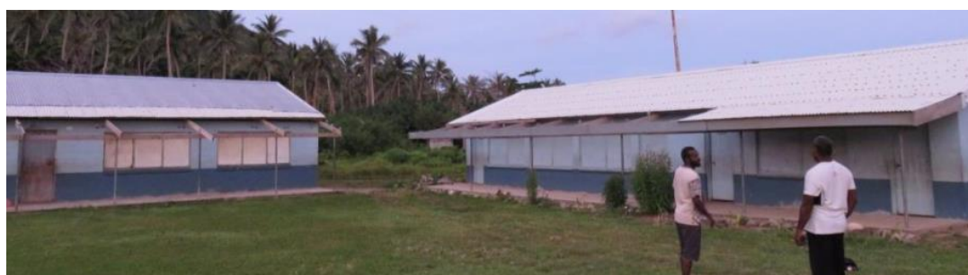
The picture above shows the two buildings in Nofo school that are to be rehabilitated by replacing the existing roofs and support structures. Photo: IFRC
