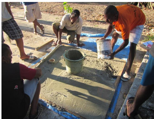
In Emae Island, Vanuatu, community members participate in the construction of pit latrines and learn how to make the base slab structure. Photo: Sofia Lardies/ New Zealand Red Cross
