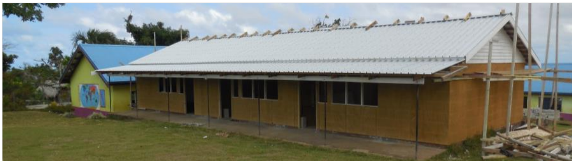
The picture above shows the Eratap school being rehabilitated. Before the rehabilitation work started, the community has contributed to the process by cleaning the site and removing all remaining roof and wall linings from the structure. Photo: IFRC
