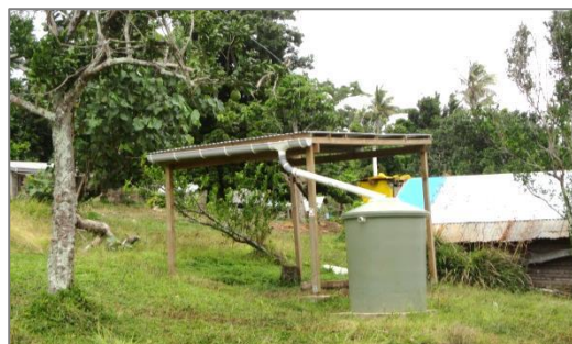
Rainwater collection system built in Sasake community, Emae. Photo: New Zealand Red Cross
