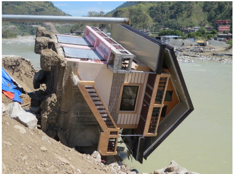
A house alongside a river in Mt. Province is toppled after the soil eroded when the river overflowed during the peak of Typhoon Haima. Photo/PRC
