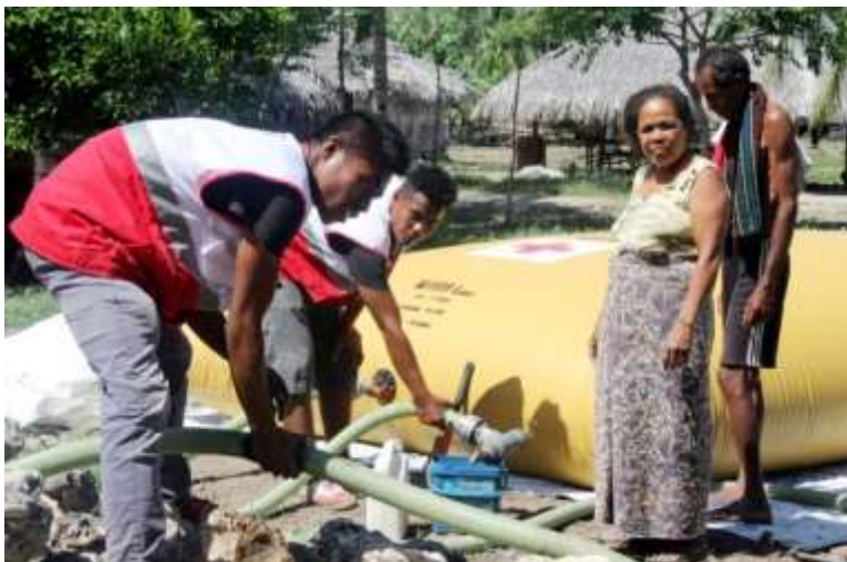
Community water distribution in Werumata Village, Bacau District (Photo: CVTL)
