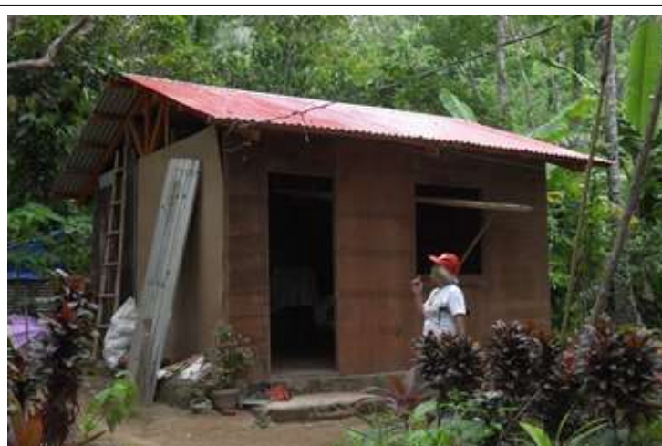
A member of the Barangay Recovery Committee monitors the completion of a repaired shelter in Santa Magdalena, Sorsogon province.
