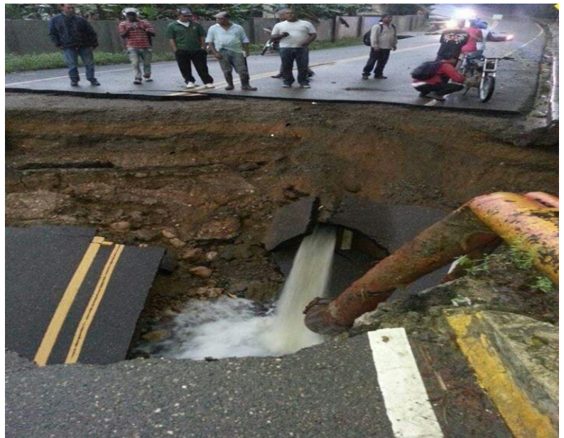
Collapsed road in the province of Espaillat in Jamaica in the north. Source: Dominican Red Cross
