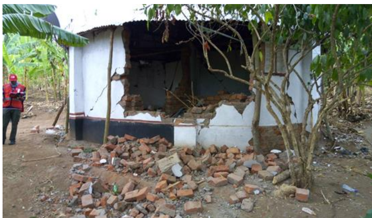
Impact of earthquake and TRCS volunteer during assessment. Picture: Stanley Nyaga
