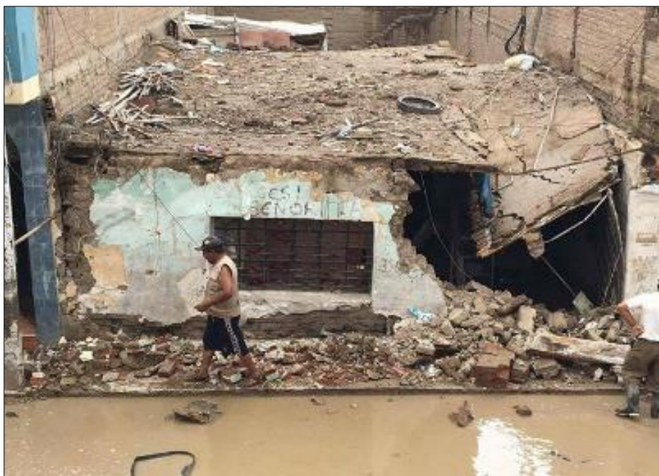
House destroyed by flooding in Lambayeque. Source: Peruvian Red Cross.
