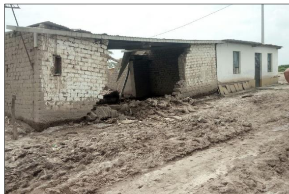
Collapsed house in the community of Jose Leonardo Ortiz in the province of Chiclayo due to flooding. Source: PRC
