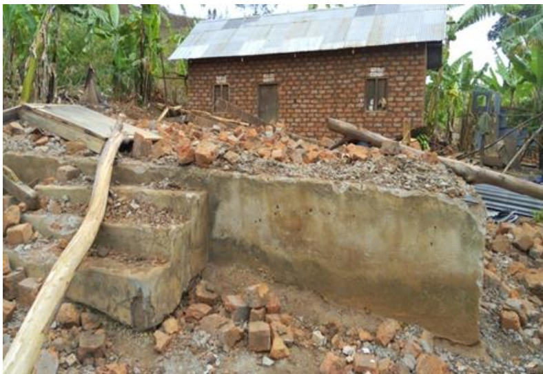
A house quickly built by a single mother of four to replace the one completely destroyed. Photo: Mukwecheni/IFRC
