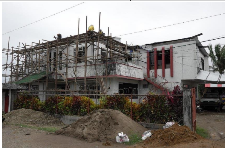
The Northern Samar chapter office was damaged due by Typhoon Nona. This operation has supported rehabilitation of the building.
