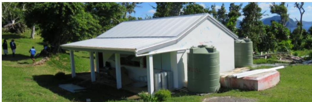
Outside view of Buninga Senecol primary school in Buninga Island close to completion, May 2016. Photo: IFRC
