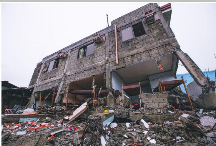
This pension house in Surigao City toppled down following the 6.7 magnitude earthquake on 10 February 2017. Aftershocks continue to be felt by many families, inducing trauma and stress to the affected population. Photo: Rommel Cabrera/IFRC
