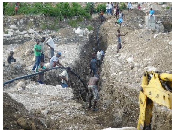
HRCS volunteers worked hand in gloves with community members in Les Coteaux to rehabilitate the Water distribution system. Source: Netherlands Red Cross
