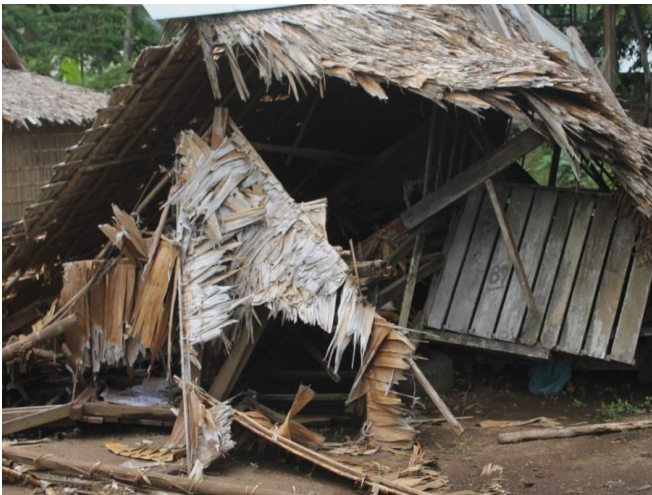
A destroyed house in Makira (photo credit: SIRC)
