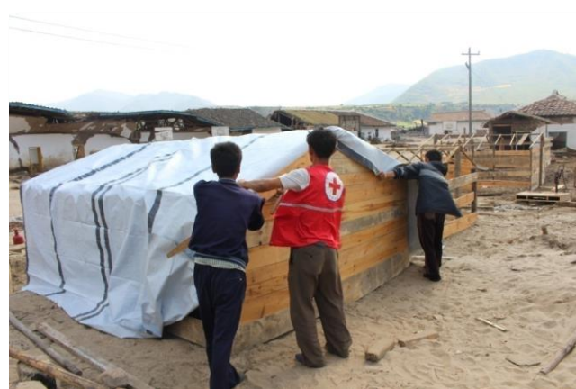
DPRK RCS's volunteers are being supported to local community for construction of Emergency Shelter (Photo: Hoeryong City Branch/DPRK RC)
