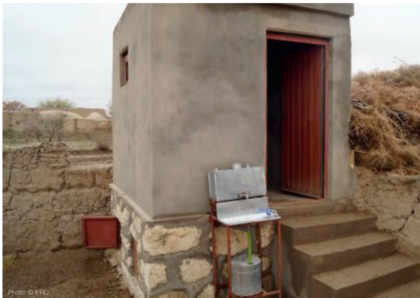
Model latrine with composting and hand-washing facilities as installed by ARCS.
