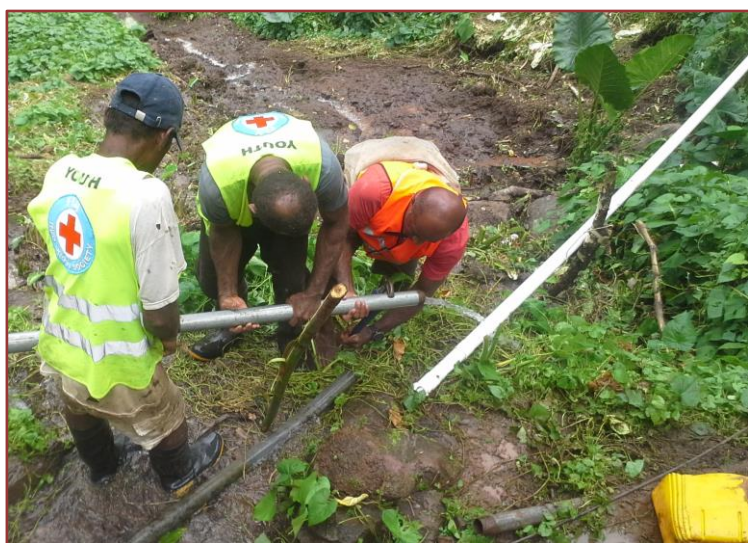
Fiji Red Cross Branch and Community Members construction of the Tuatua Village in Koro Island for safe water supply to the community members. January, 2017
