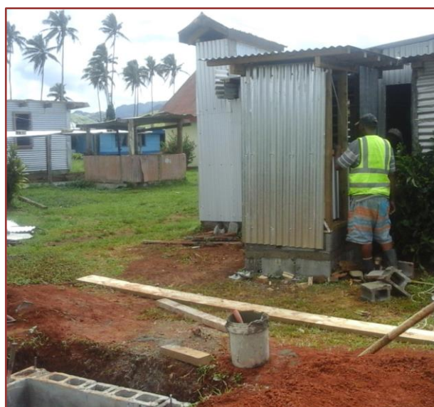
Fiji Red Cross and Community members constructing a single household latrine in Ra. April, 2017
