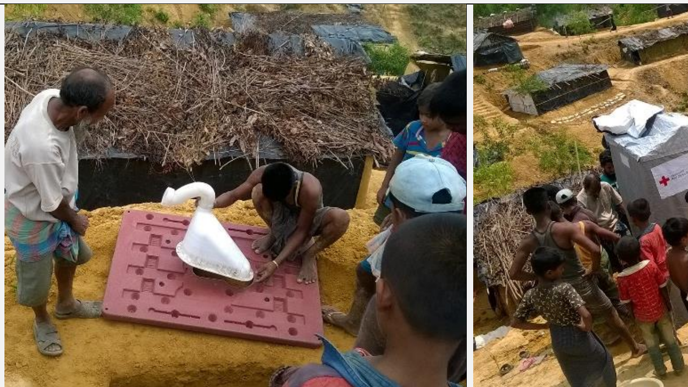
With BDRCS support, community managed to install mobile latrines in the Kutupalong and Balukhali makeshift camp. (Photo: Arafat/NDWRT Member, BDRCS)
