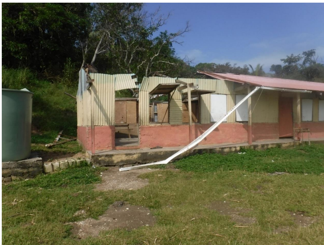
Damaged school in Malekula (Photo: VRCS)
