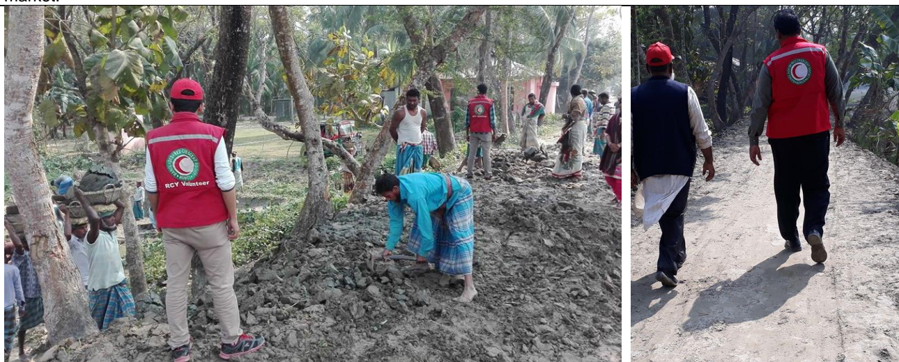
With the support of community people, BDRCS was repairing the damaged road in Lakshmipur district. (Photo: BDRCS)
