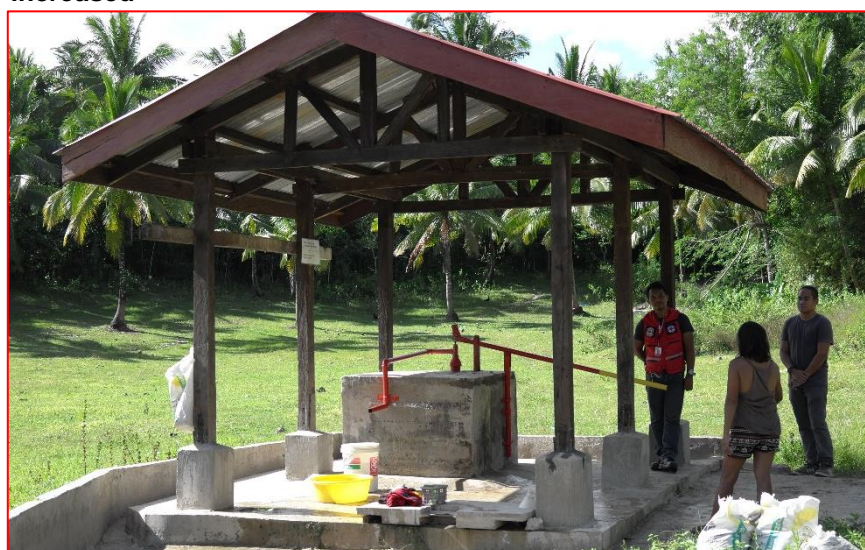
A water-source installed in Tabuelan, Cebu province through the support of the WASH programme of PRC and IFRC. Photo: IFRC
