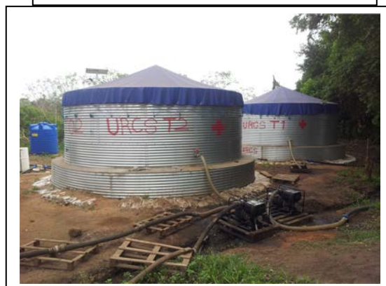
Figure 3. URCS Water Treatment Unit Enyau (Source: IFRC WASH Coordinator)
