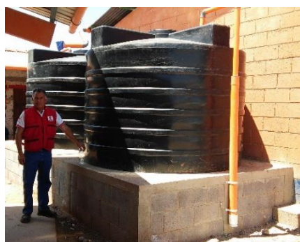
Photo: San Francisco School - 2017 School rainwater collection and storage system. Source: GRC
