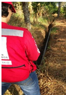
Photo: Quiché delegation 2016. PVC pipe for potable water conduction. Source: GRC
