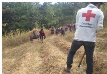
Photo: Quiché delegation, 2016. Terrace construction for soil conservation in Choyomche III. Source: GRC
