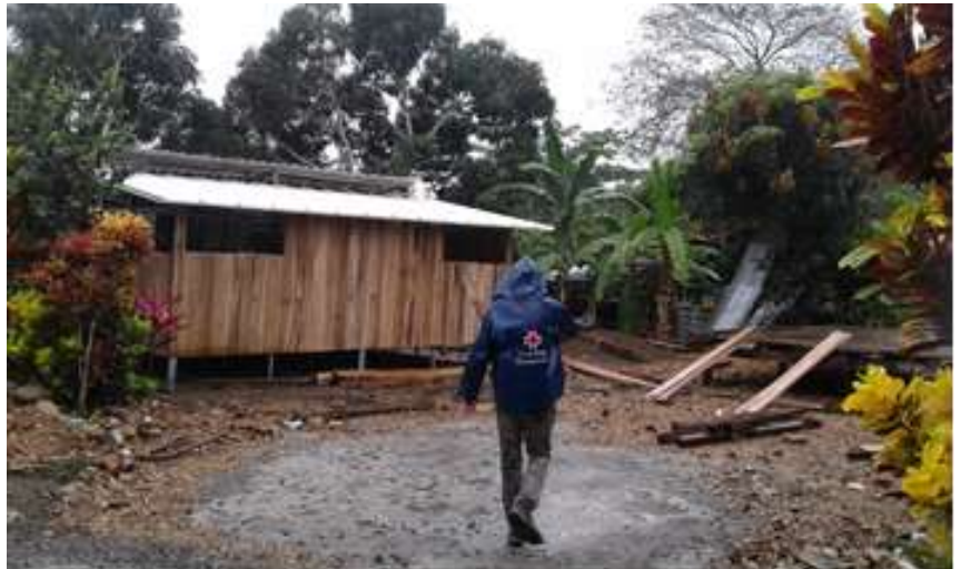
The Ecuadorian Red Cross has provided permanent housing solutions in prioritized communities. Source: ERC
