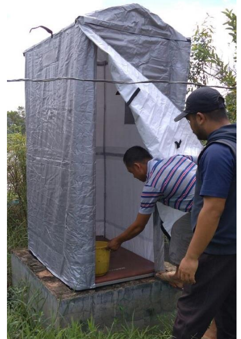
IRCS volunteers erecting a temporary toilet in a flood affected area of Manipur, (Photo: IRCS)
