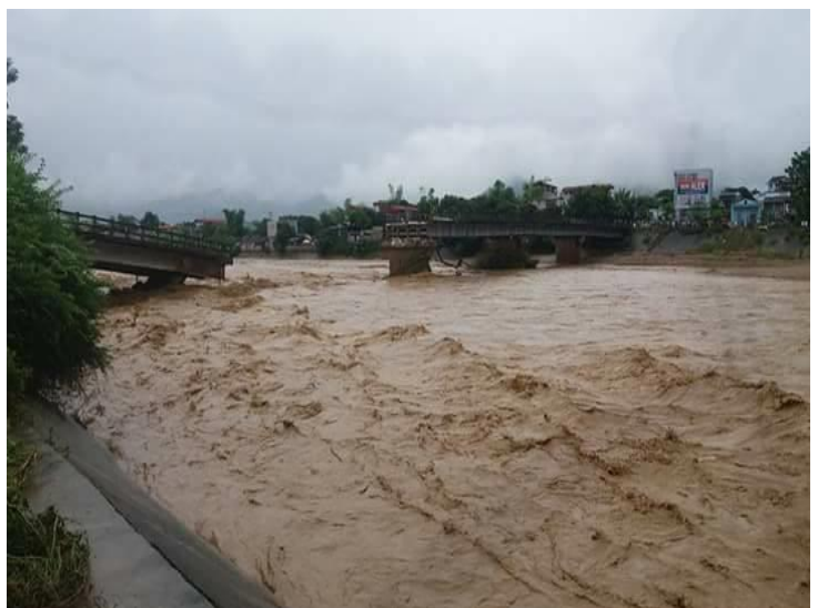
Broken Thia Bridge in Nghia Lo, Yen Bai province
